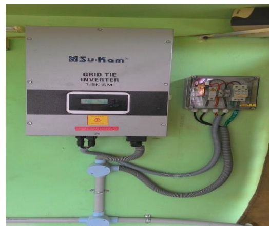
Fig. 3. (c) solar grid inverter
