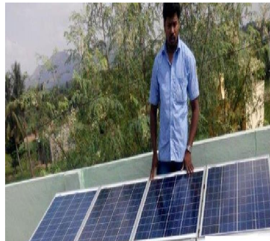
Fig. 3. (a) solar photovoltaic panel array
