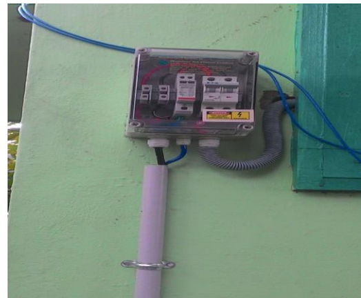
Fig. 3. (b) DC distribution box
